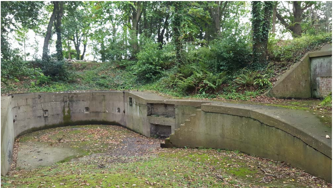
Emplacement for 9inch HA. Ammunition issue hatch on the extreme right. Photo (C) Steve Berden
