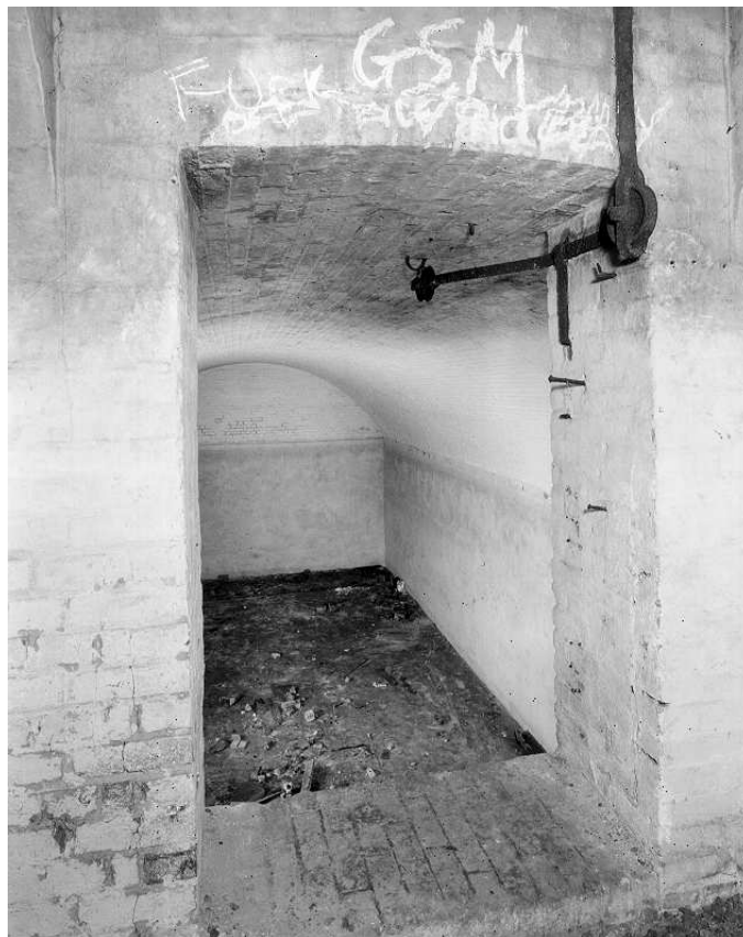
Figure 29 No 2 water tank, with the pulley in the foreground (NMR: AA00/9837)
